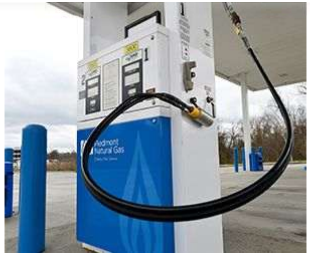
Natural gas vehicle refueling station
